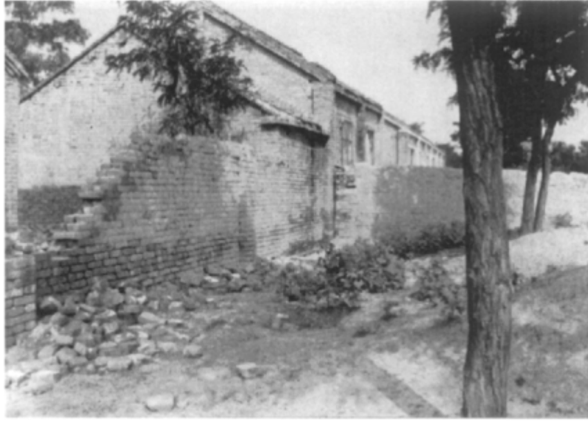
Schoolhouse in need of repair
